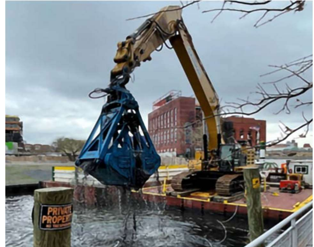
Excavator removing sediment from Gowanus Canal between Carroll and 3 rd Street bridges
