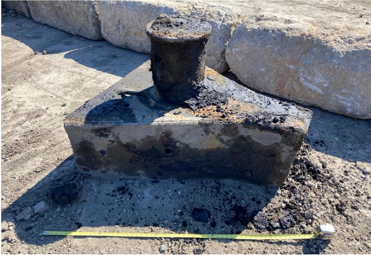
Photograph 1 – View of bollard item, front view.
