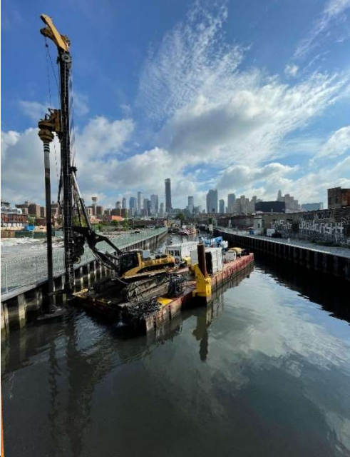
Contractors adding cement mix to canal bottom using drilling equipment mounted on barges.
