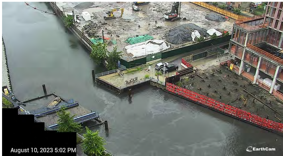
Figure 8. Sheen and turbid discharge from high level storm sewer pipe on August 10, 2023 at 5:00 PM.
