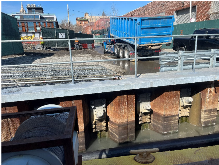
Figure 8. Turbid discharge on February 27, 2023 at 10:45 AM from truck wash activities on DeGraw Street associated with upland construction activities.
