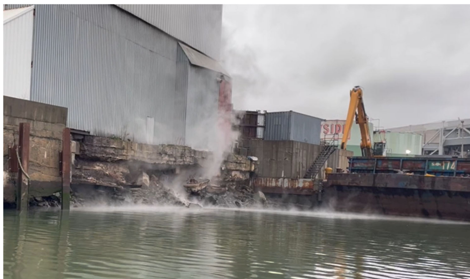
Figure 8. Discharge from concrete plant on March 14, 2023 at 8:45 AM.
