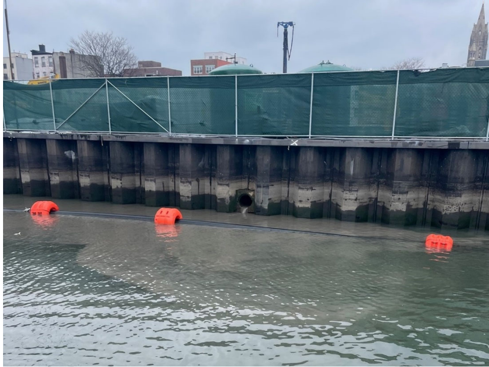
Figure 9. Turbid discharge from the storm water outfall at the Bayside North construction site located between Union Street and Degraw Street on March 23, 2023 at 1:30 PM.
