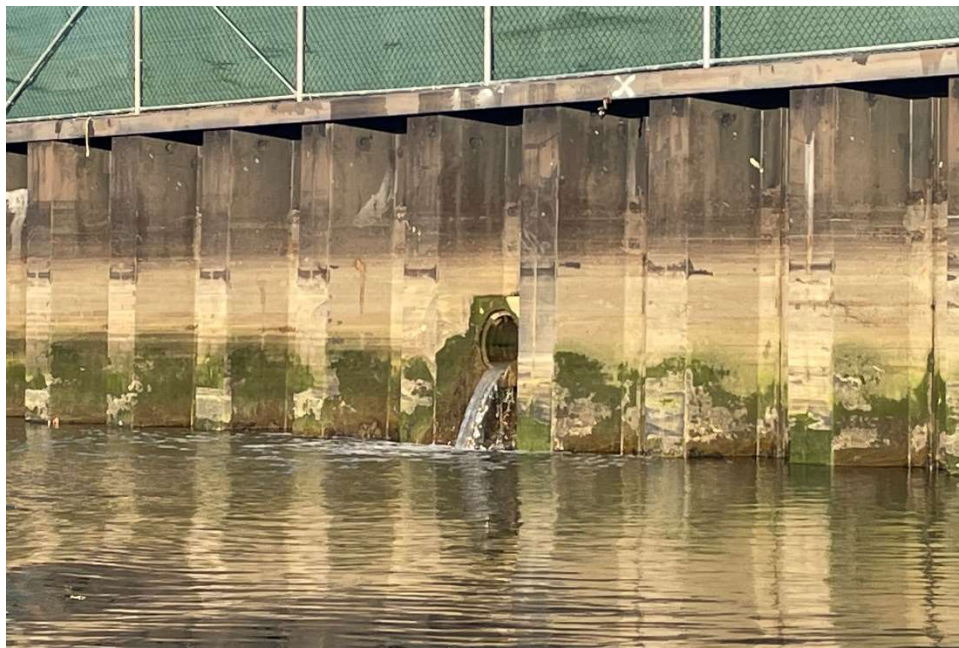
Figure 7. Turbid discharge from the storm water outfall at the Bayside North construction site located between Union Street and Degraw Street on March 27, 2023 at 7:45 AM.
