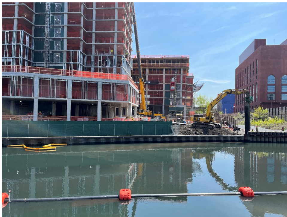
Figure 11. Turbid discharge from southwest corner of 420 Carroll on April 20, 2023 at 11:45 AM.
