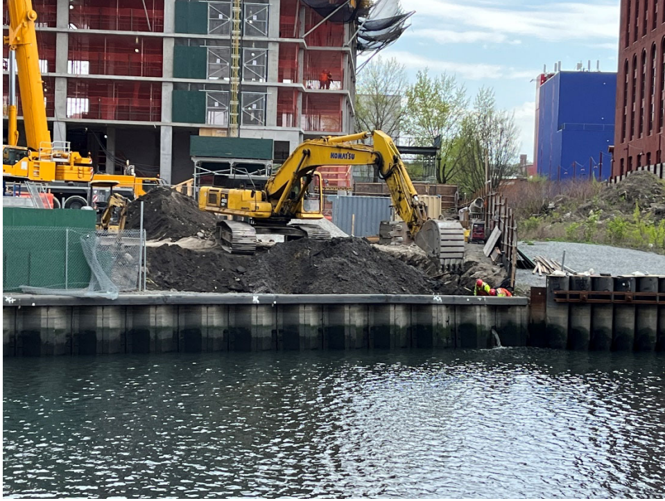
Figure 8. Discharge from southwest corner of 420 Carroll on April 18, 2023 at 11:30 AM.
