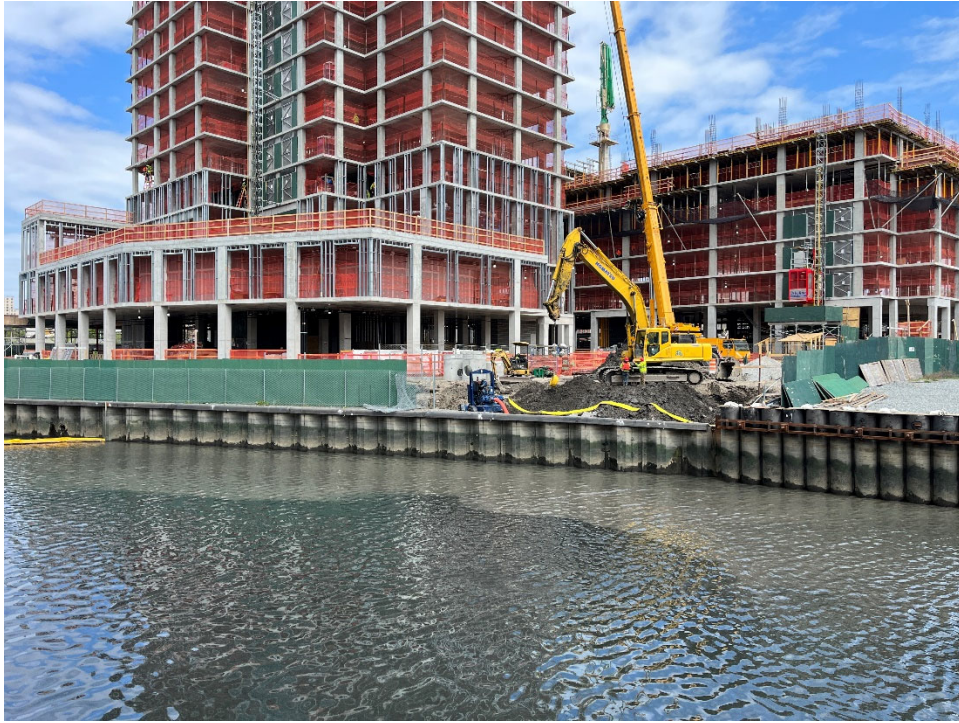
Figure 9. Turbid discharge from southwest corner of 420 Carroll on April 18, 2023 at 2:15 PM.
