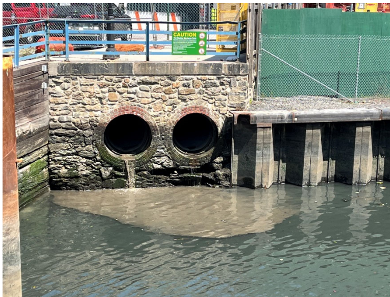
Figure 8. Turbid discharge from the high level storm sewer pipe on May 18, 2023 at 2:30 PM.
