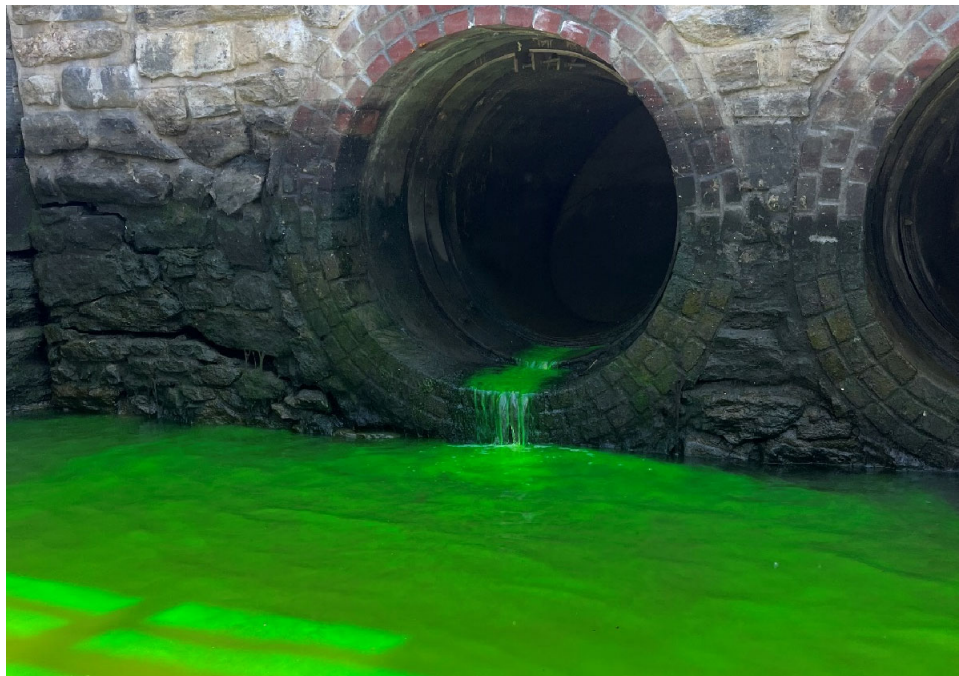
Figure 6. Discharge of suspected dye tracer test from high level storm sewer pipe on June 2, 2023 at 10:45 AM.
