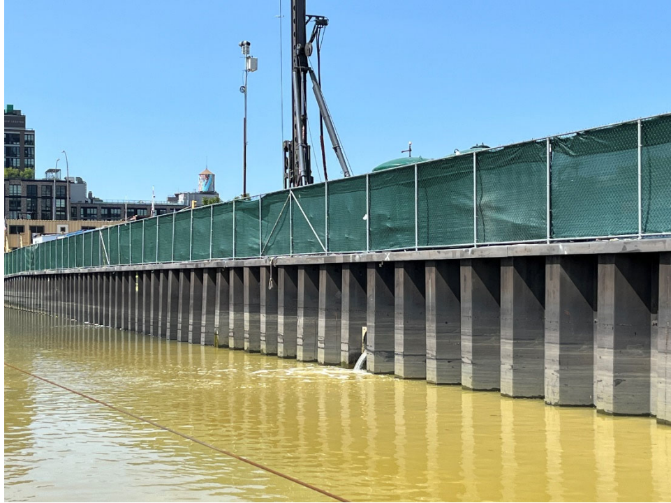
Figure 7. Discharge from the storm water outfall at the Bayside North construction site located between Union Street and Degraw Street on May 30, 2023 at 11:00 AM.
