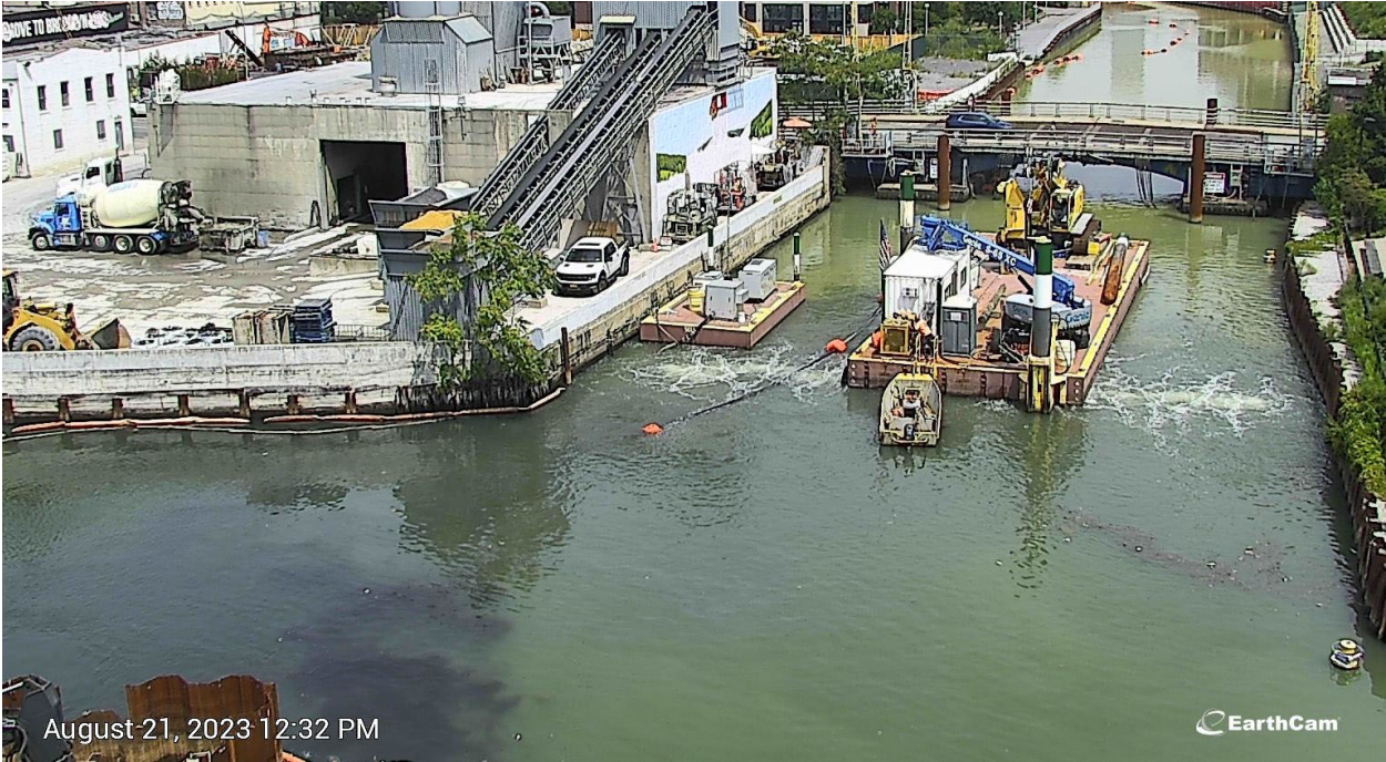
Figure 11. Turbid discharge from the Salt Lot on August 21, 2023 at 12:30 PM.
