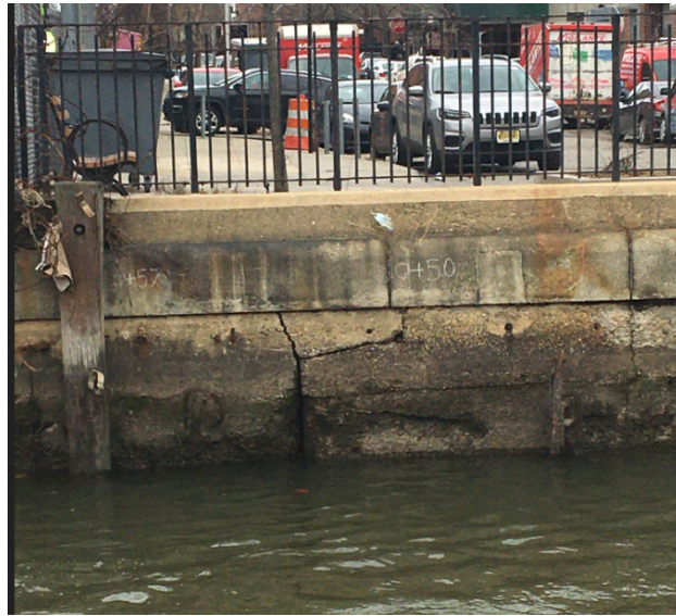
Figure 7. Crack at Douglass Street concrete slab above
