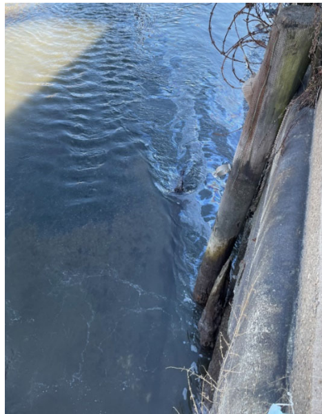
Figure 8. Sheen from the crack at Douglass Street
