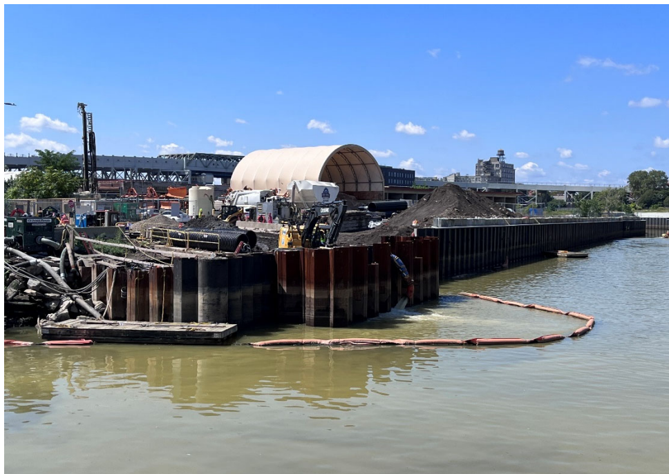
Figure 11. Turbid discharge from the Salt Lot on August 30, 2023 at 12:45 PM.
