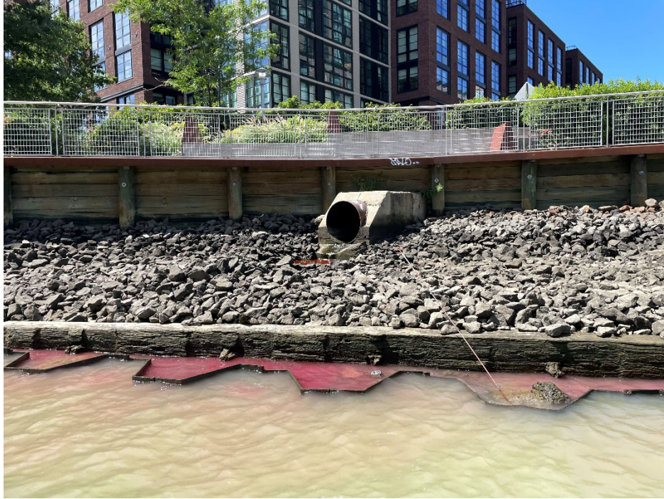
Figure 8. Red discharge from storm drain at Bond Street Promenade on August 31, 2023 at 1:00 PM.
