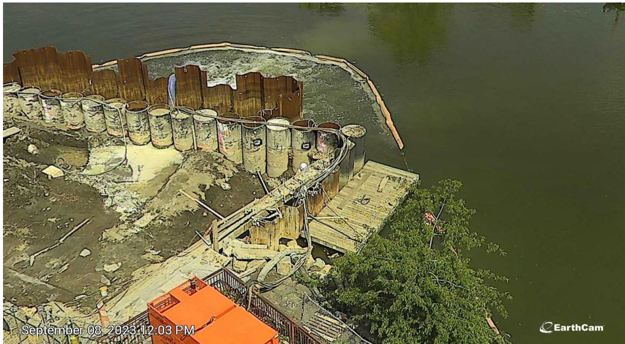
Figure 10. Turbid discharge from the Salt Lot on September 8, 2023 at 12:00 PM.
