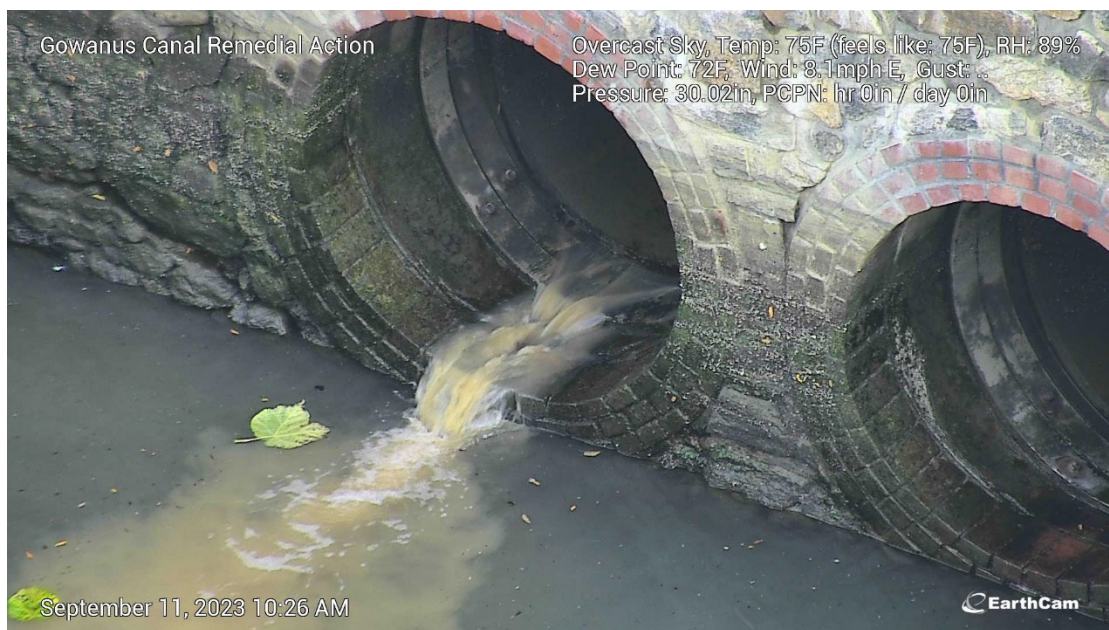
Figure 7. Discharge from high level storm sewer pipe on September 11, 2023 at 10:30 AM.
