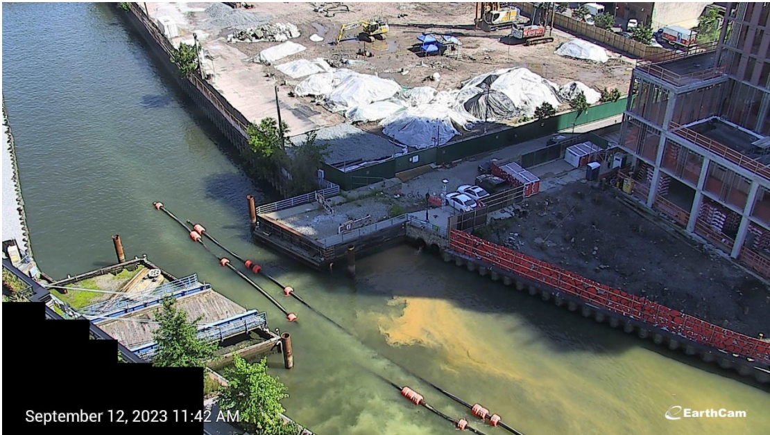
Figure 9. Discharge from high level storm sewer pipe on September 12, 2023 at 11:45 AM.
