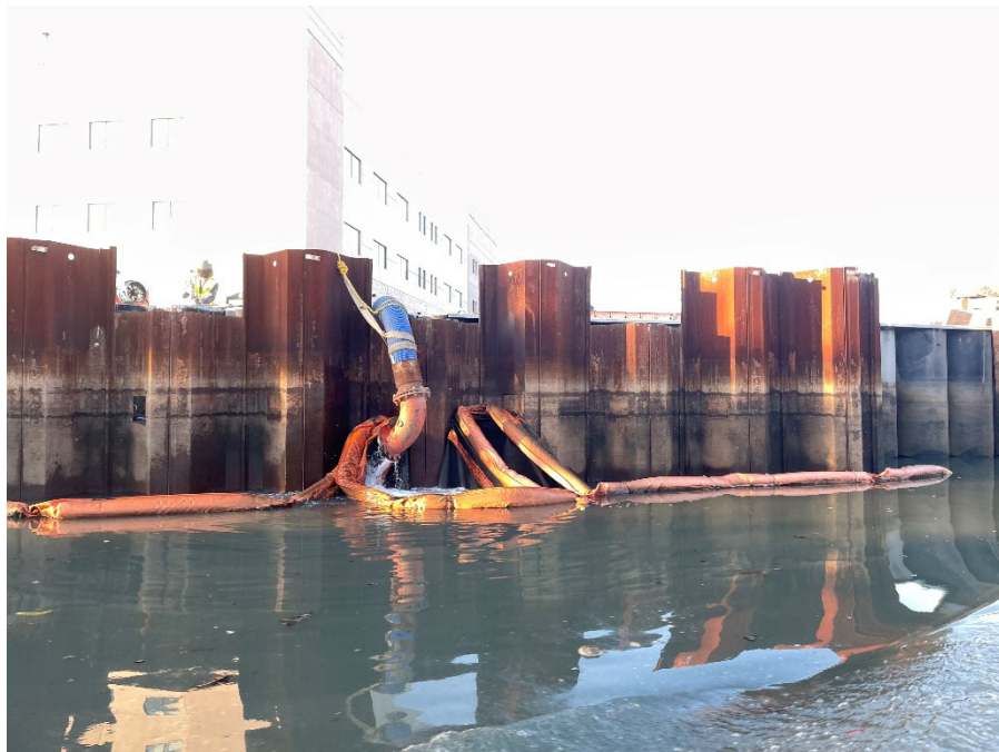
Figure 10. Turbid discharge from the Salt Lot cofferdam on September 21, 2023 at 7:30 AM.
