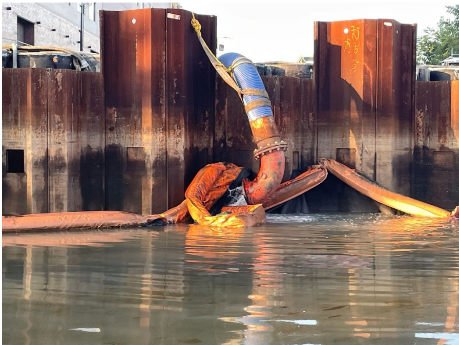
Figure 9. Turbid discharge from the Salt Lot cofferdam on September 19, 2023 at 7:30 AM.
