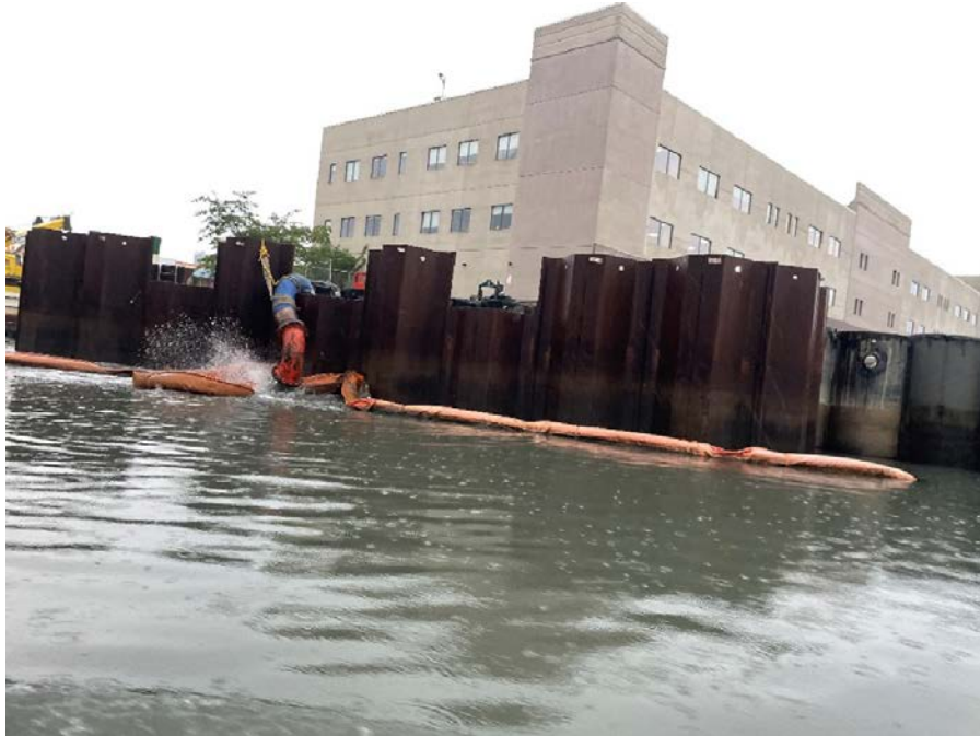
Figure 8. Turbid discharge from the Salt Lot cofferdam on September 18, 2023 at 7:30 AM.
