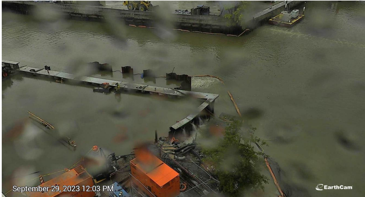
Figure 10. Turbid discharge from the Salt Lot cofferdam on September 29, 2023 at 12:00 PM.
