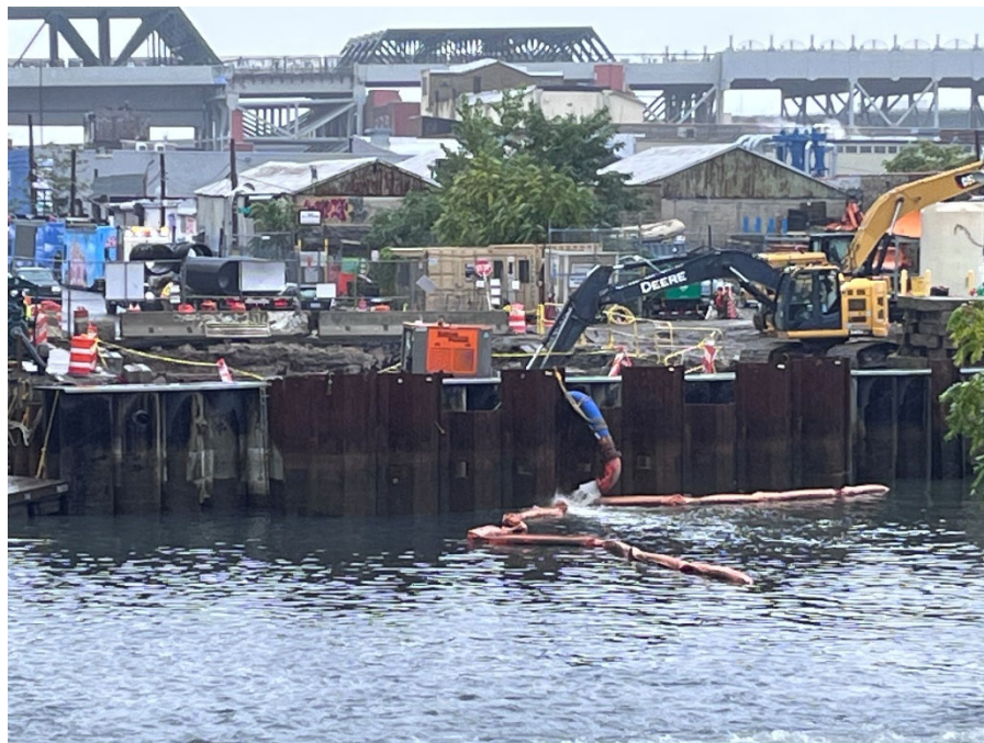
Figure 11. Turbid discharge from the Salt Lot cofferdam on September 25, 2023 at 10:45 AM.
