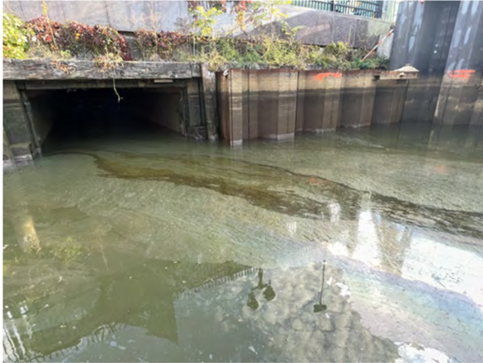
Figure 8. Sheen discharge from headwall CSO at 9:00 AM on October 24, 2023.
