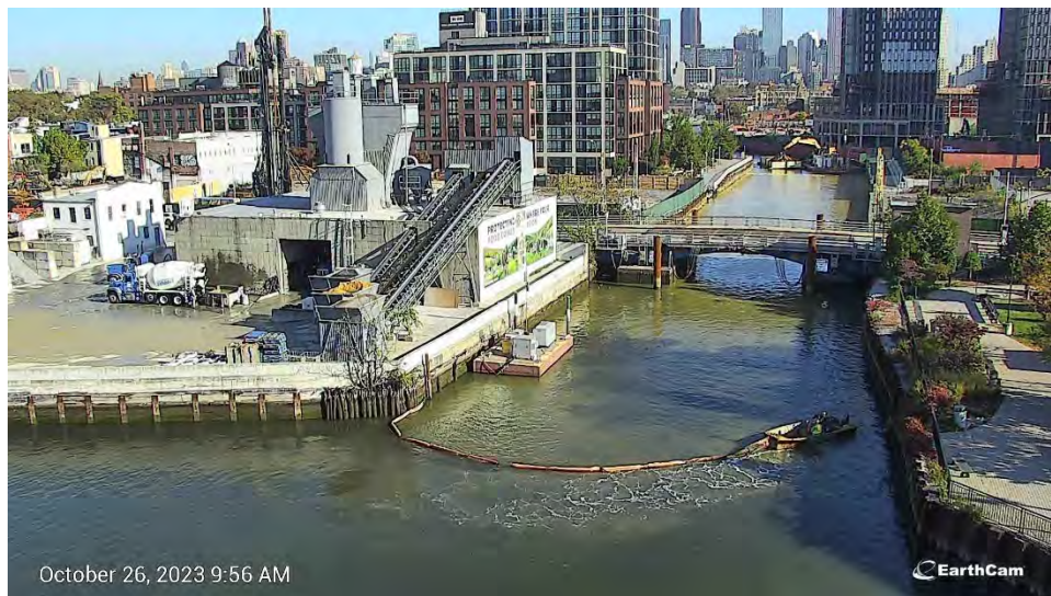
Figure 7. Turbidity curtain being installed south of the Third Street Bridge at 10:00 AM on Thursday, October 26, 2023.
