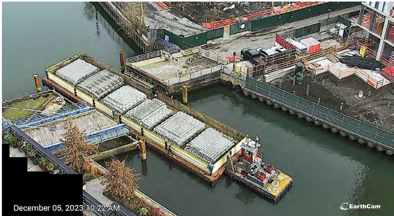
Figure 9. Vessel transporting a double mini-hopper loaded with ACB Mats through Carroll Street Bridge on December 5, 2023 at 10:15 AM.
