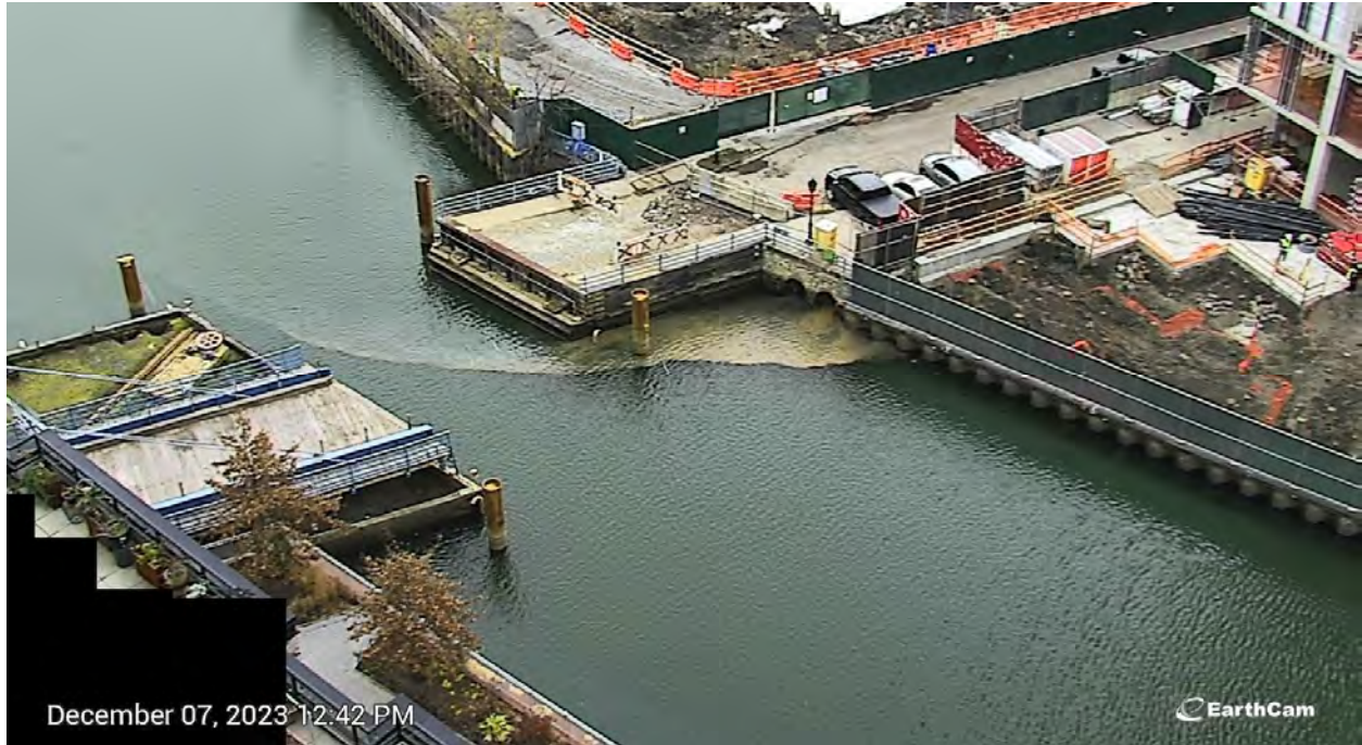
Figure 8. Turbid discharge from the high-level storm sewer pipe adjacent to OH-005 on December 7, 2023 at 12:45 PM.
