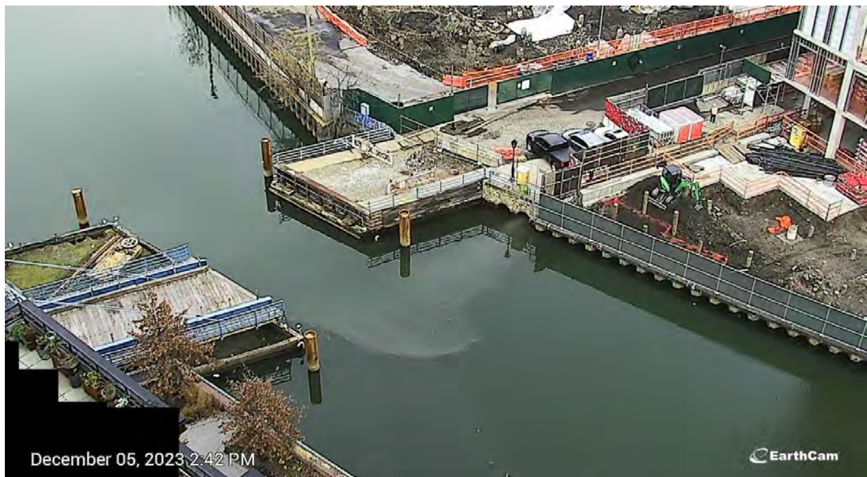
Figure 7. Turbid discharge from the high-level storm sewer pipe adjacent to OH-005 on December 5, 2023 at 2:45 PM.
