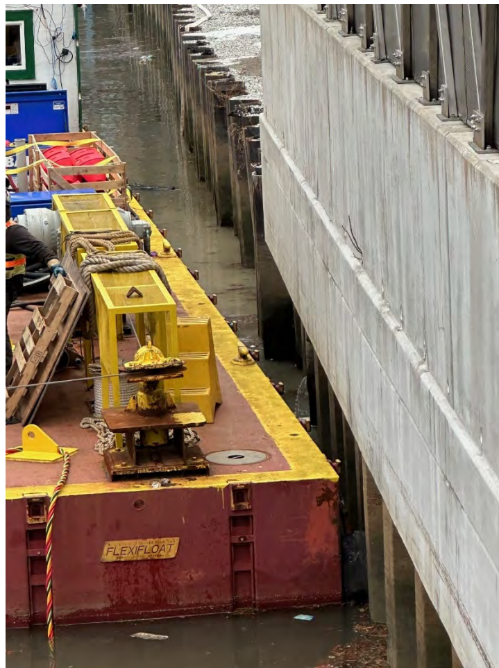
Figure 7. Discharge related to a concrete pour at the northern Presidents Street property on Wednesday, January 10, 2024.
