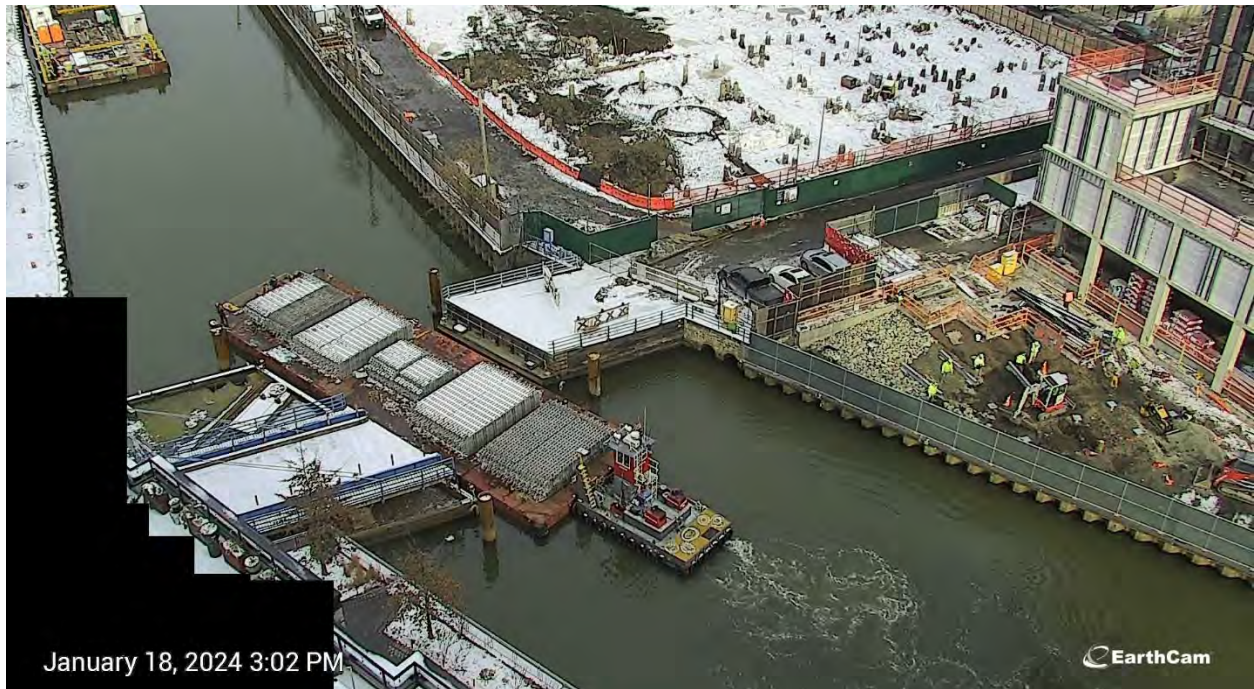
Figure 8. Vessel transporting a barge loaded with ACB Mats through Carroll Street Bridge at approximately 3:00 PM on January 18, 2024.
