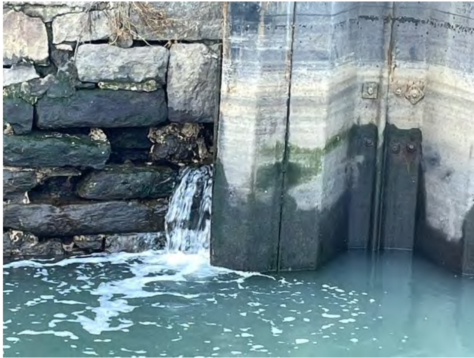
Figure 12. Discharge from between the sheetpile bulkhead of the 383 Carroll Street property and the stone bulkhead at Carroll Street Bridge, observed the morning of February 7, 2024.
