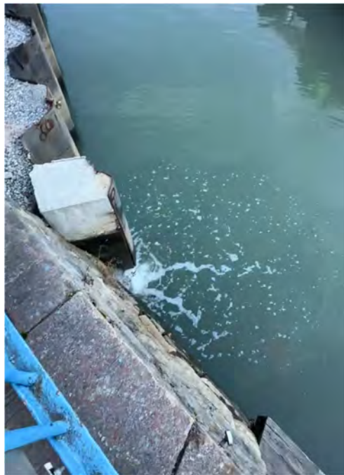
Figure 11. Discharge from between the sheetpile bulkhead of the 383 Carroll Street property and the stone bulkhead at Carroll Street Bridge, observed the morning of February 7, 2024.
