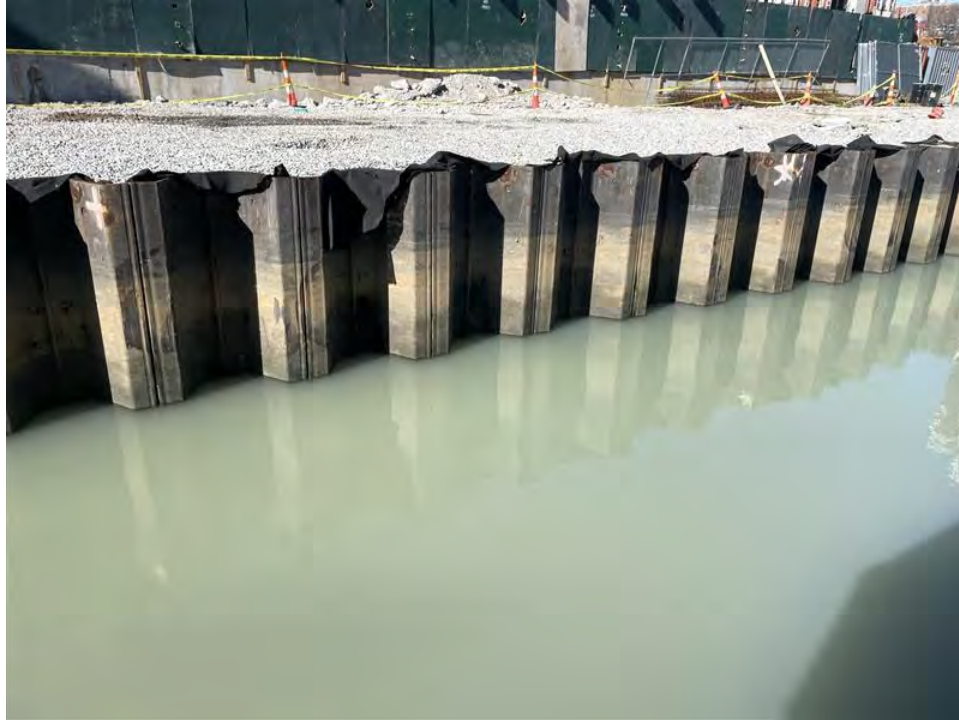
Figure 10. Observations of elevated turbidity between Carroll Street Bridge and Union Street Bridge at 12:45 PM on Tuesday, February 6, 2024 at 12:00 PM.
