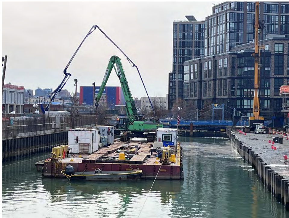
Figure 13. Surface foam generated during grout placement for structural concrete and CLSM installation in the middle pool (i.e. between Union Street Bridge and Carroll Street Bridge), observed on Monday of the reporting period.
