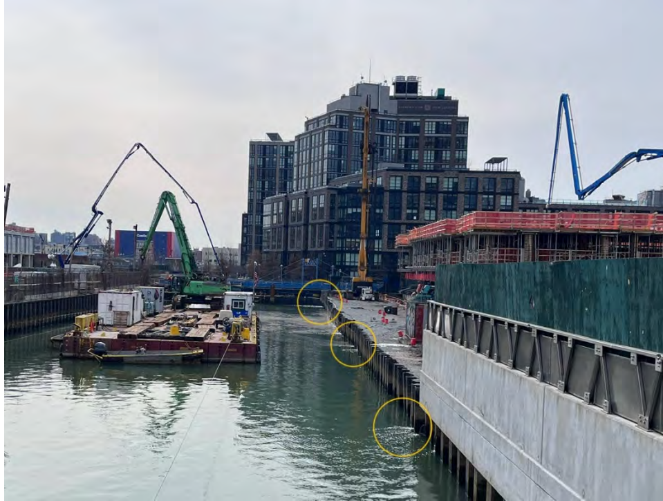
Figure 12. Additional discharges from the 383 Carroll Street property sheetpiles, observed Monday of the reporting period.
