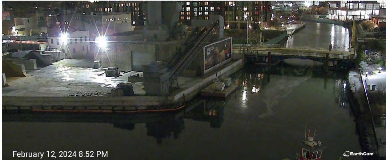
Figure 7. Visual action level exceedance south of Third Street Bridge was observed on Monday evening of the reporting period, when a northerly wind pushed the surface foam (related to CLSM/structural concrete installation) south and outside of RTA1.
