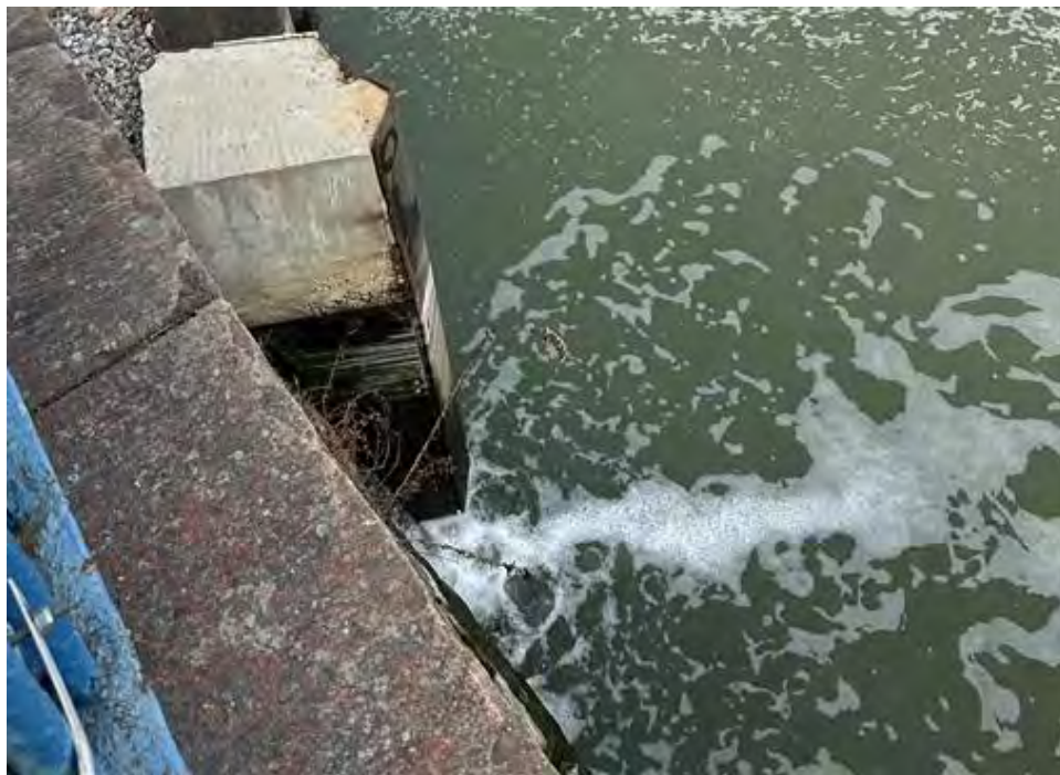
Figure 12. Discharge from between the sheetpile bulkhead of the 383 Carroll Street property and the stone abutment at Carroll Street Bridge, observed Monday of the reporting period.
