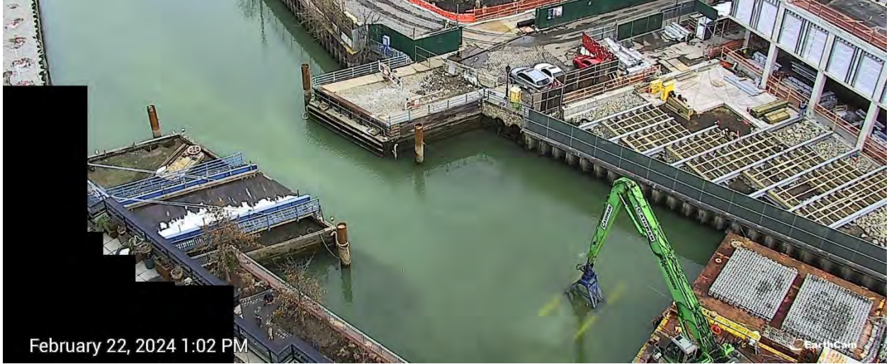
Figure 15. Observations of the Thursday, February 22, 2024, turbidity event were continuously documented throughout the day. Turbidity was confined to RTA1 and migrated as far south as the northern portion of the south pool (south of Carroll Street Bridge).
