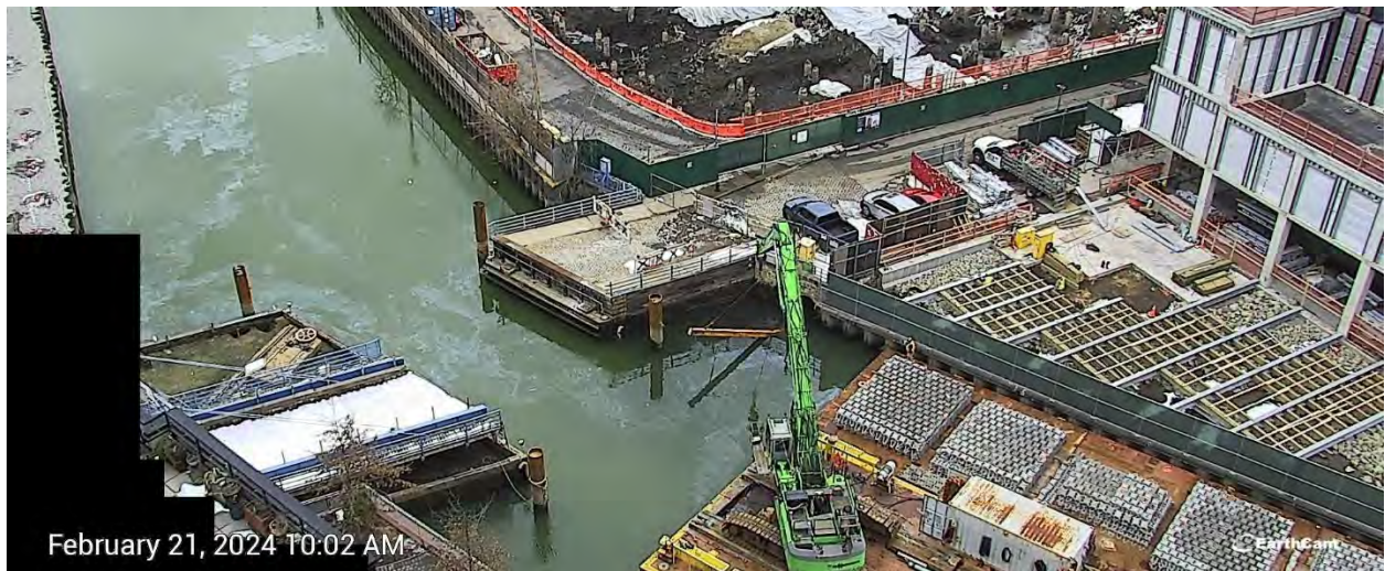
Figure 8. Observations of the Wednesday, February 21, 2024, sheen event were continuously documented throughout the day. The sheen was confined to the middle pool (between Union Street Bridge and Carroll Street Bridge) and the northern portion of the south pool (south of Carroll Street Bridge).
