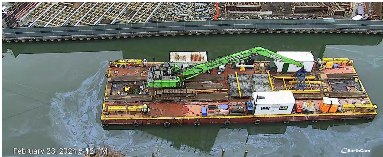
Figure 12. Observations of the Friday, February 23, 2024, sheen event were continuously documented throughout the day. The sheen was confined to the middle pool (between Union Street Bridge and Carroll Street Bridge) and the northern portion of the south pool (south of Carroll Street Bridge).
