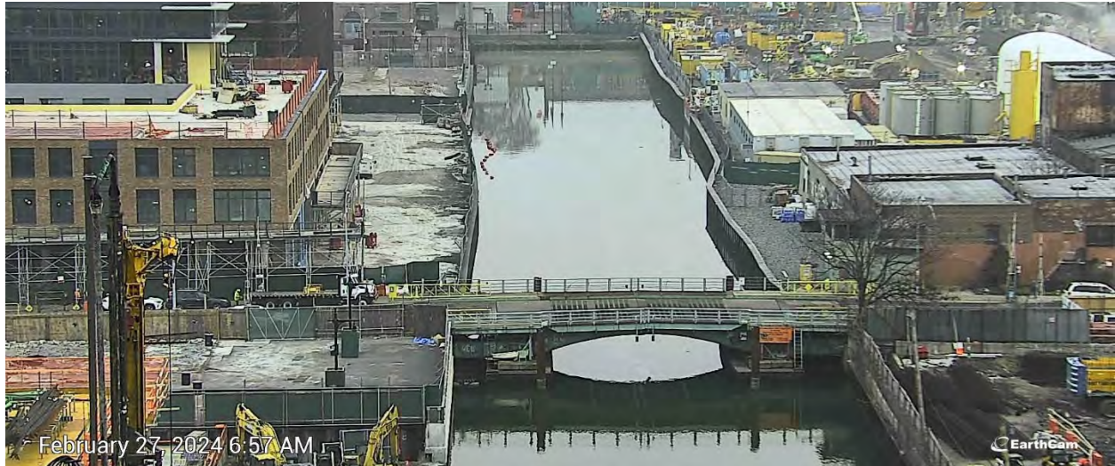
Figure 9. At 7:00 AM on Tuesday, February 27, 2024, a sheen was observed north of Union Street Bridge migrating south with a northeasterly wind and an incoming tide (prior to any remedial construction activities).
