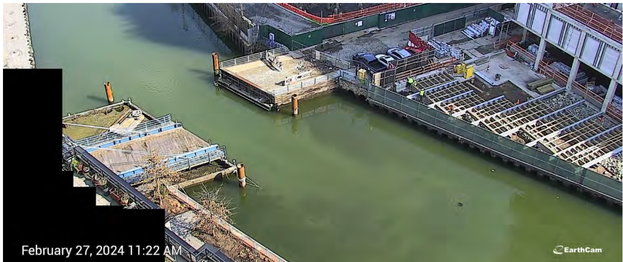
Figure 12. At 11:30 AM on Tuesday, February 27, 2024, turbidity unrelated to remedial construction activities was observed migrating south in the middle and south pools with a northeasterly wind and an outgoing tide. The turbidity was confined to RTA1.
