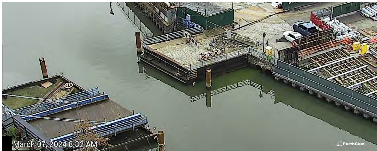
Figure 11. Turbid discharge from high level storm sewer pipe on March 7, 2024 at 8:30 AM.
