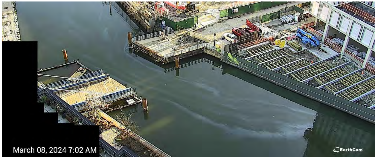
Figure 12. At 7:00 AM on Friday, March 5, 2024, a sheen was observed around Street Bridge migrating south with a northeasterly wind and an outgoing tide (prior to any remedial construction activities).
