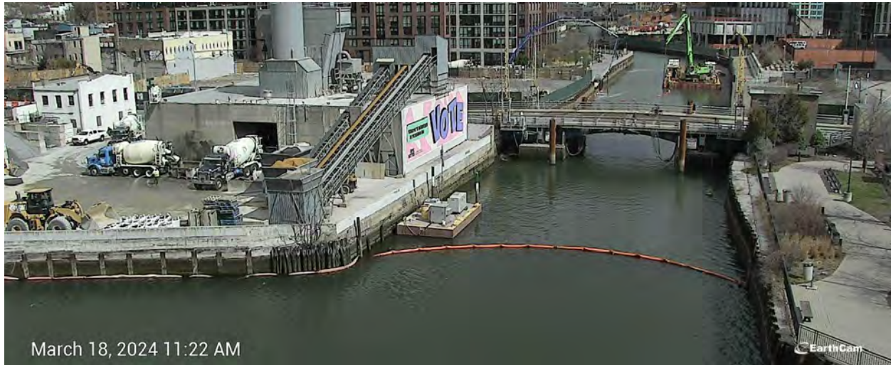
Figure 7. Turbidity curtain installed south of the Third Street Bridge on Monday, March 18, 2024.
