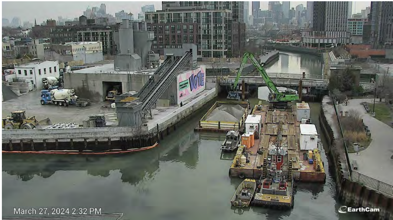
Figure 12. Visual indication of elevated turbidity as a result of gravel placement in and around Third Street Bridge and temporarily suspended sediments from passing vessels at 12:15 PM on Wednesday, March 27, 2024.
