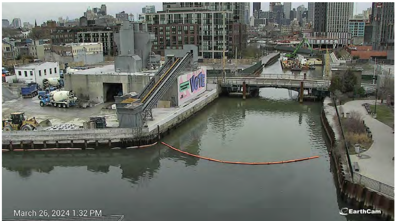
Figure 11. Turbidity curtain installed south of the Third Street Bridge at 1:30 PM on Tuesday, March 26, 2024.
