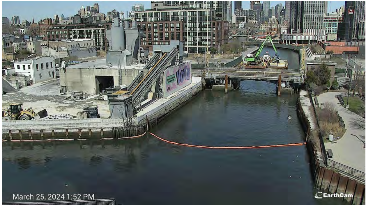
Figure 8. Turbidity curtain installed south of the Third Street Bridge at 1:45 PM on Monday, March 25, 2024.
