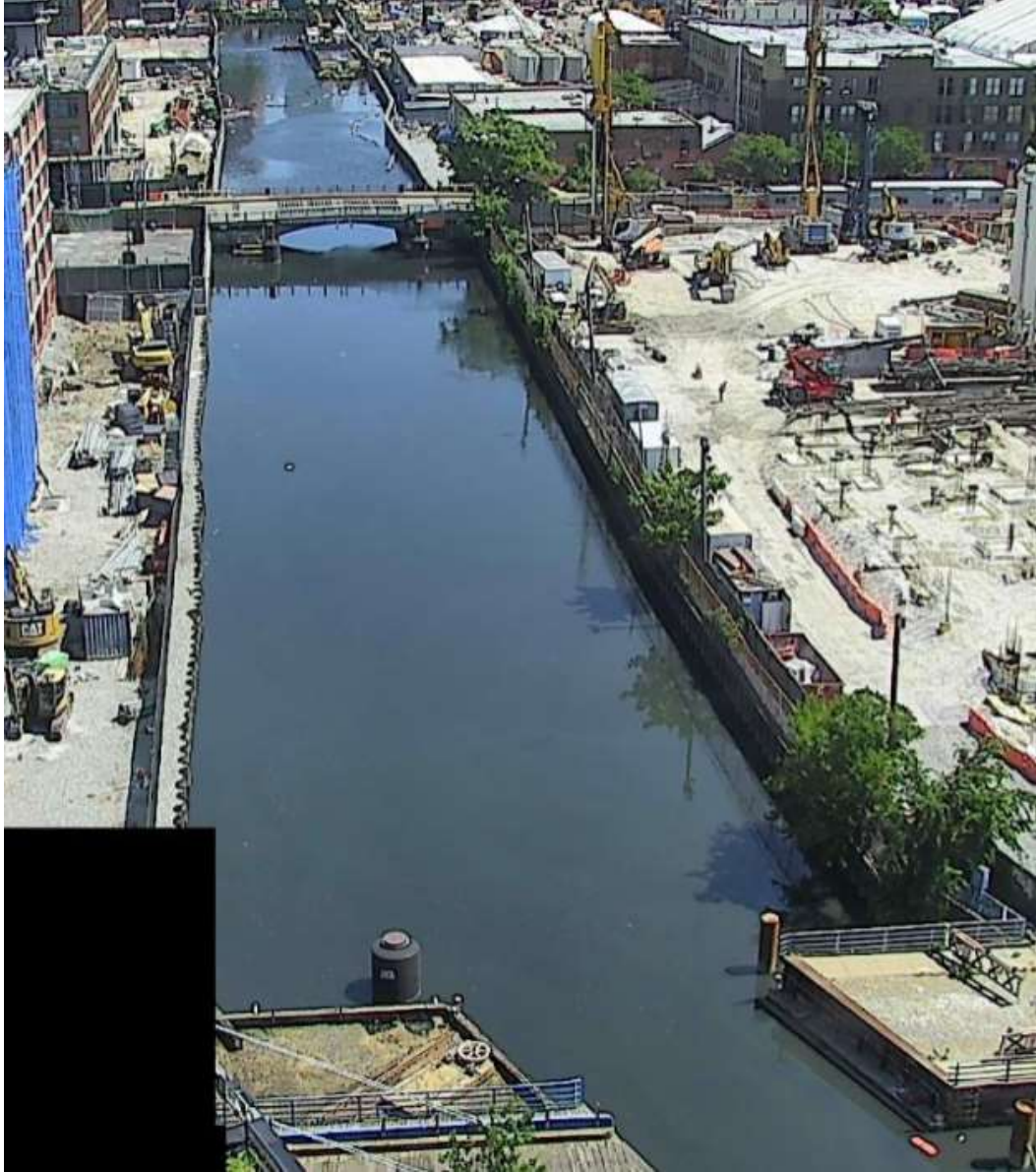
Figure 7 - June 25, 2024. Canal water with a dark coloration observed north of the 3 rd Street Bridge. Turbidity unrelated to construction activities also observed.
