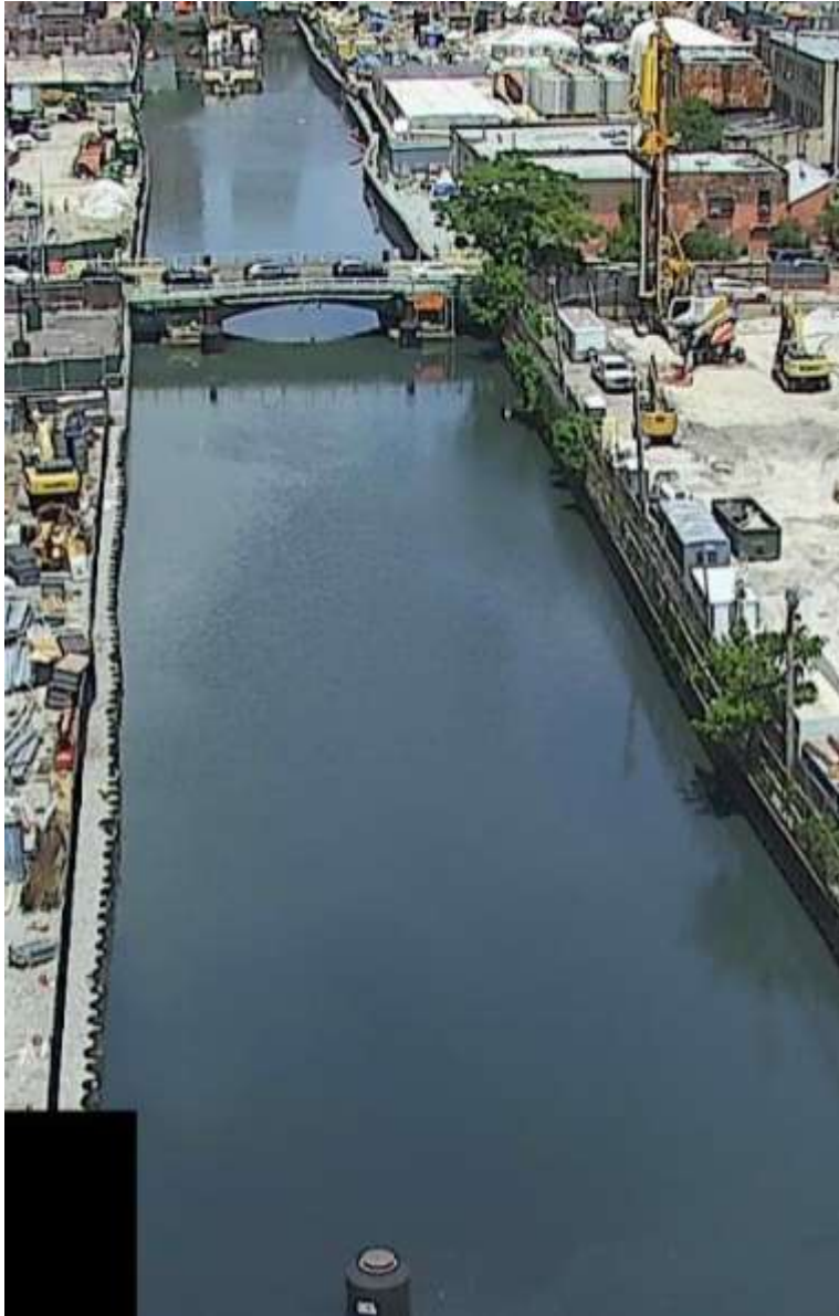
Figure 8- June 26, 2024. Canal water with a dark coloration observed north of the turbidity curtain at Station# 3+00. Turbidity unrelated to construction activities also observed.
