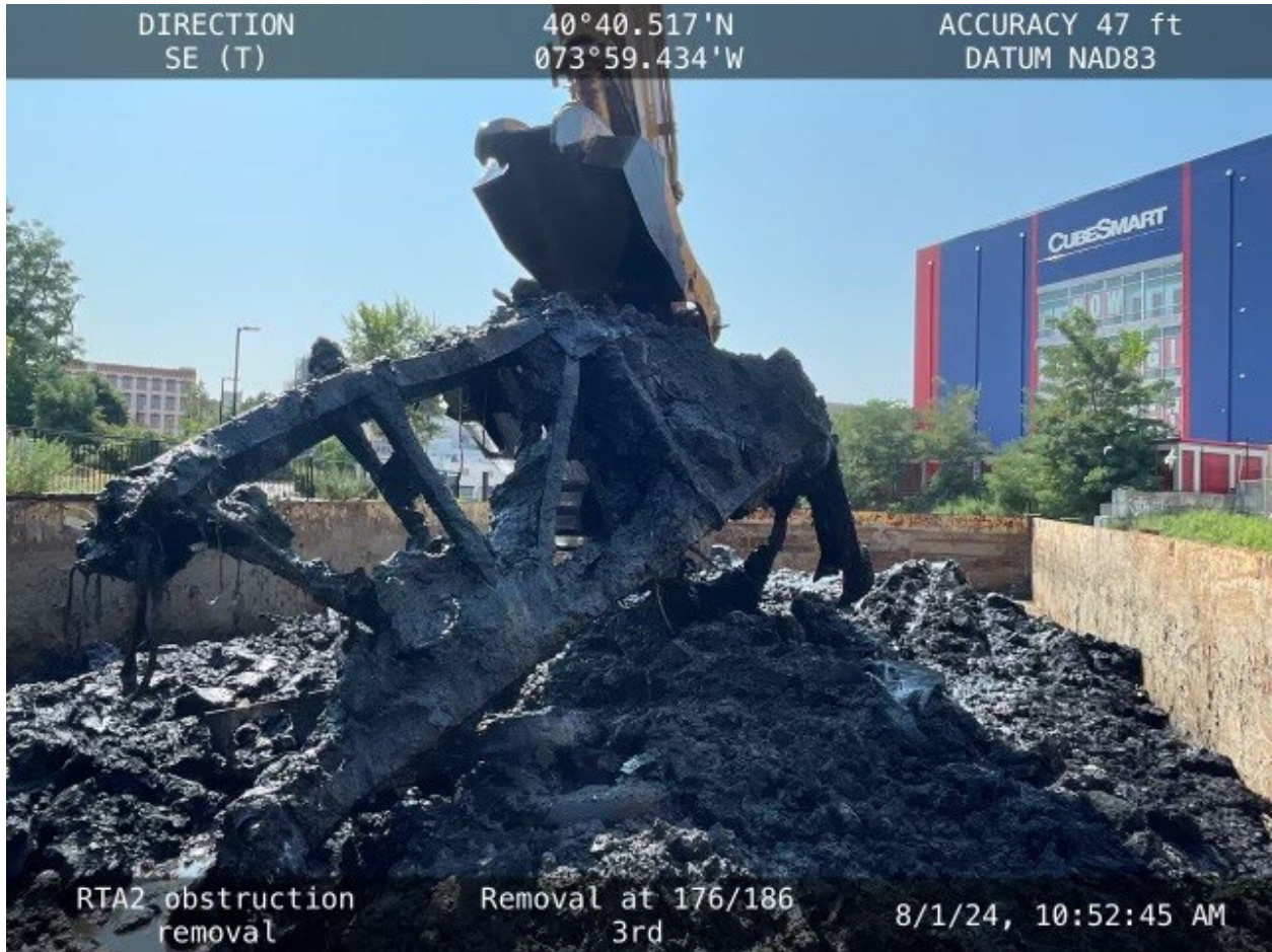
Photograph 1. Steel Truss identified in Level 1 monitoring of dredging within TB-6 (Geosyntec Consultants/GZA, August 1, 2024).
