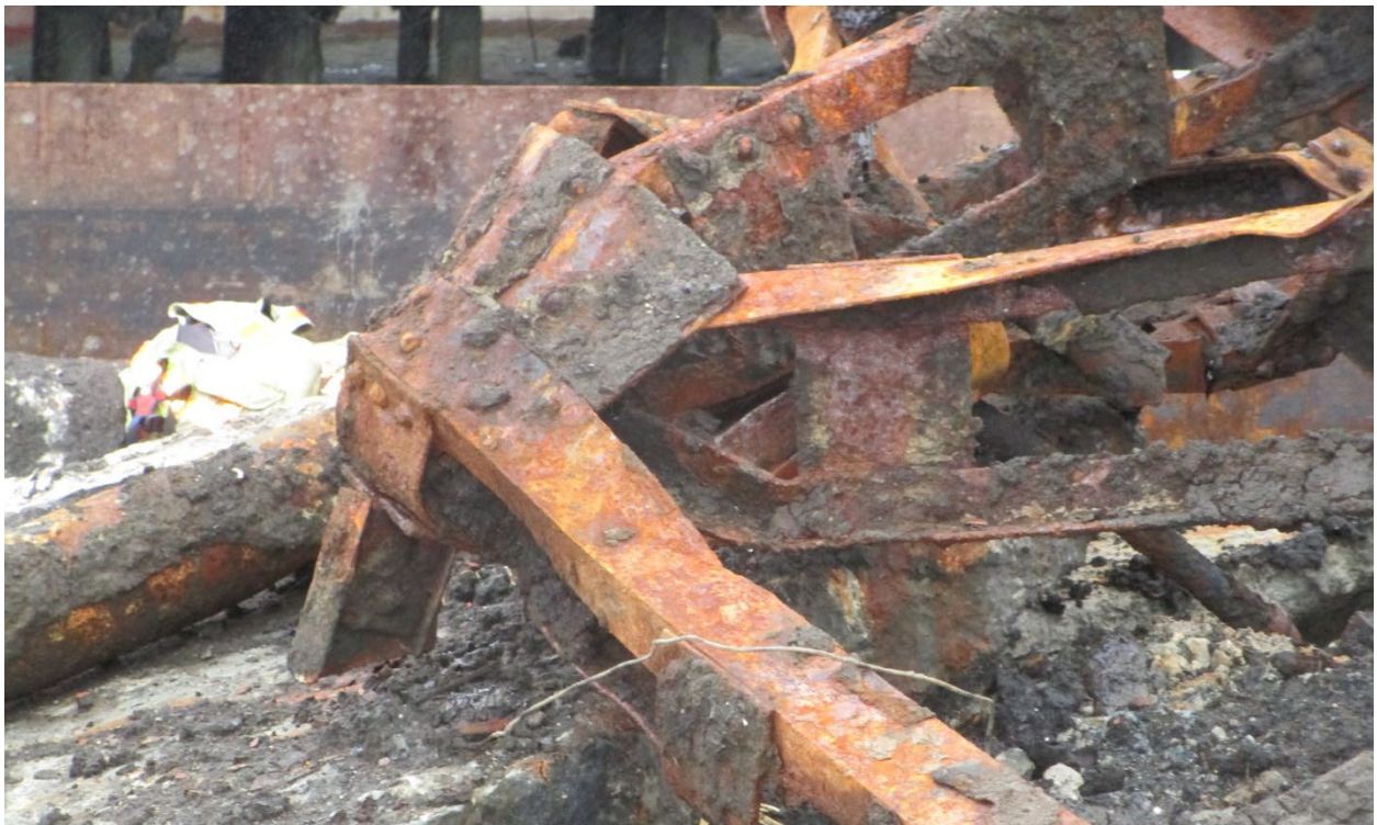
Photograph 3. Steel truss: Detail of angle iron and rivet construction (Chronicle Heritage, August 7, 2024).
