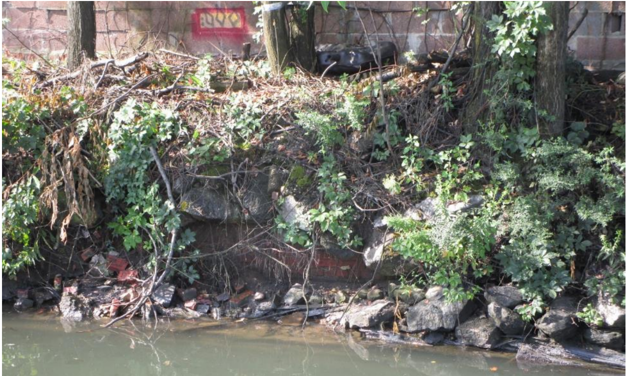
Photograph 4. Partially intact brick wall and broken concrete fragments on south wall of TB-7 in proximity of removed Target 42b. View is facing south (Chronicle Heritage, August 19, 2024).
