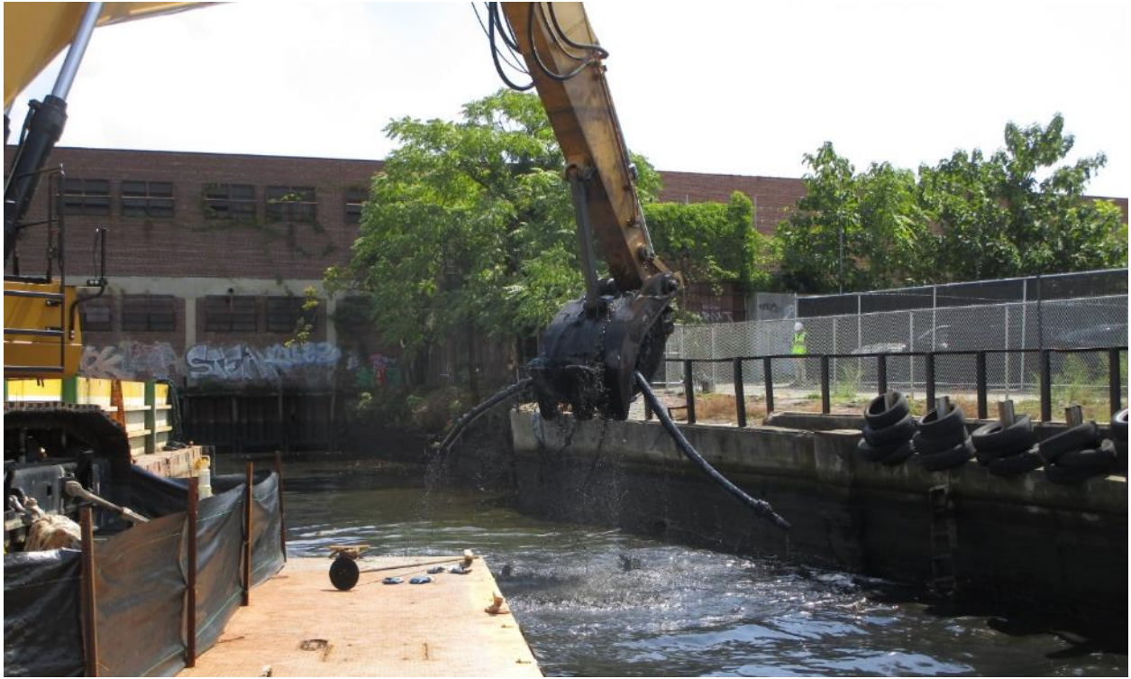
Photograph 3. Dredging of Target 42b – included removal of concrete, tires, and metal piping. View is facing southeast (Chronicle Heritage, August 19, 2024).
