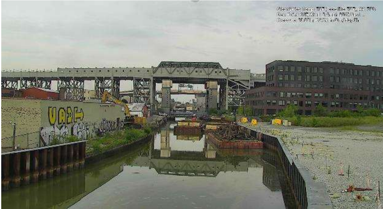
Figure 8 – July 22, 2024. General Conditions in Canal north of 9 th Street Bridge prior to work activities at 6:52AM.
