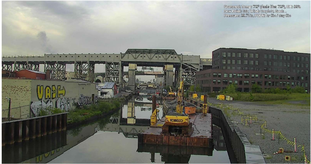
Figure 9 – August 19, 2024. General Conditions in Canal north of 9 th Street Bridge prior to work activities at 07:07. Moderate sheens noted prior to work activities.
