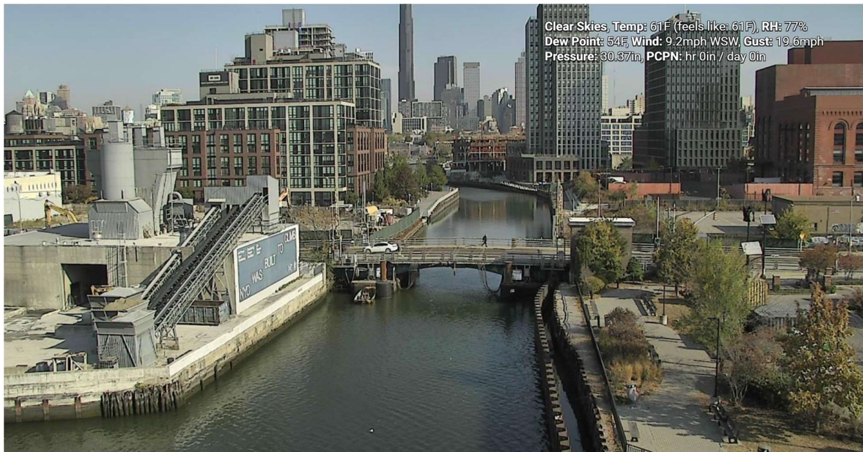
Figure 9– October 30, 2024. General Conditions in Canal south of 3 rd Street Bridge during work activities at midmorning.
