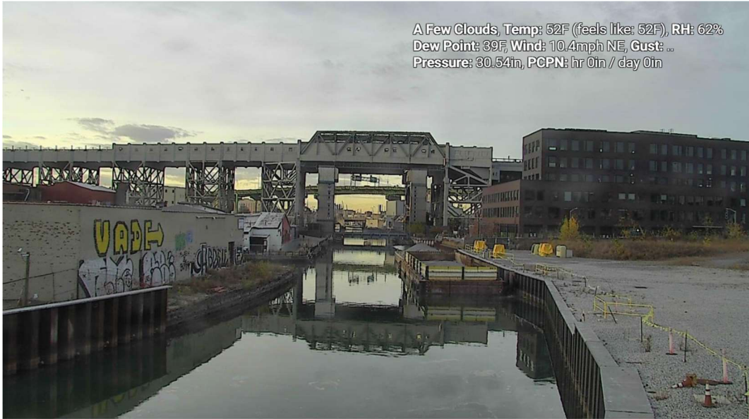
Figure 8 – November 4, 2024. General Conditions in Canal looking towards 9 th Street Bridge prior to work activities. Slight sheen noted.
