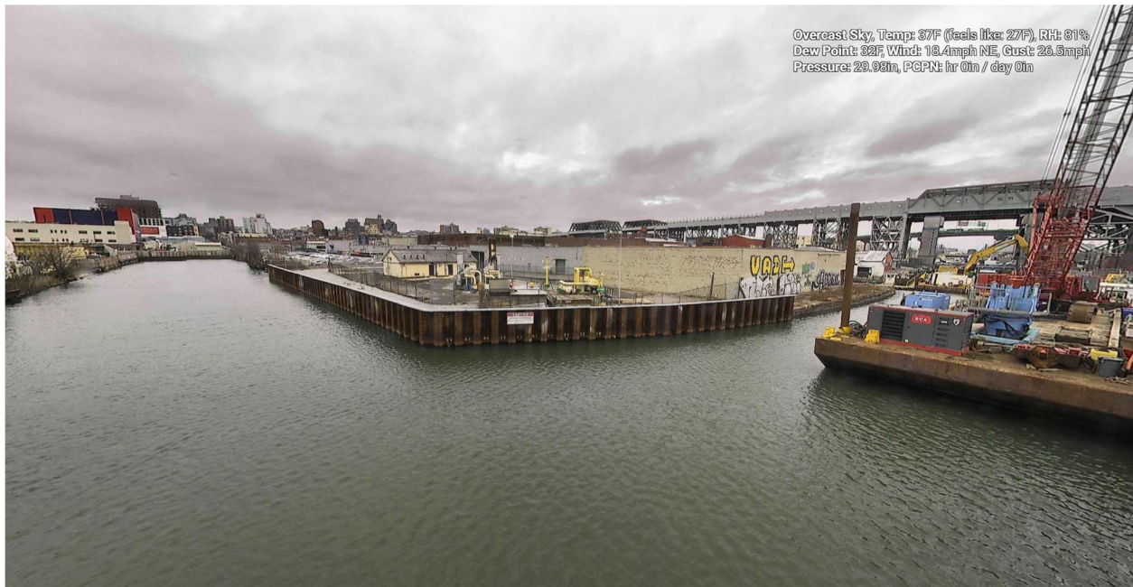
Figure 10– December 20, 2024. General Conditions in Canal north of 9 th Street Bridge during work activities work activities.
