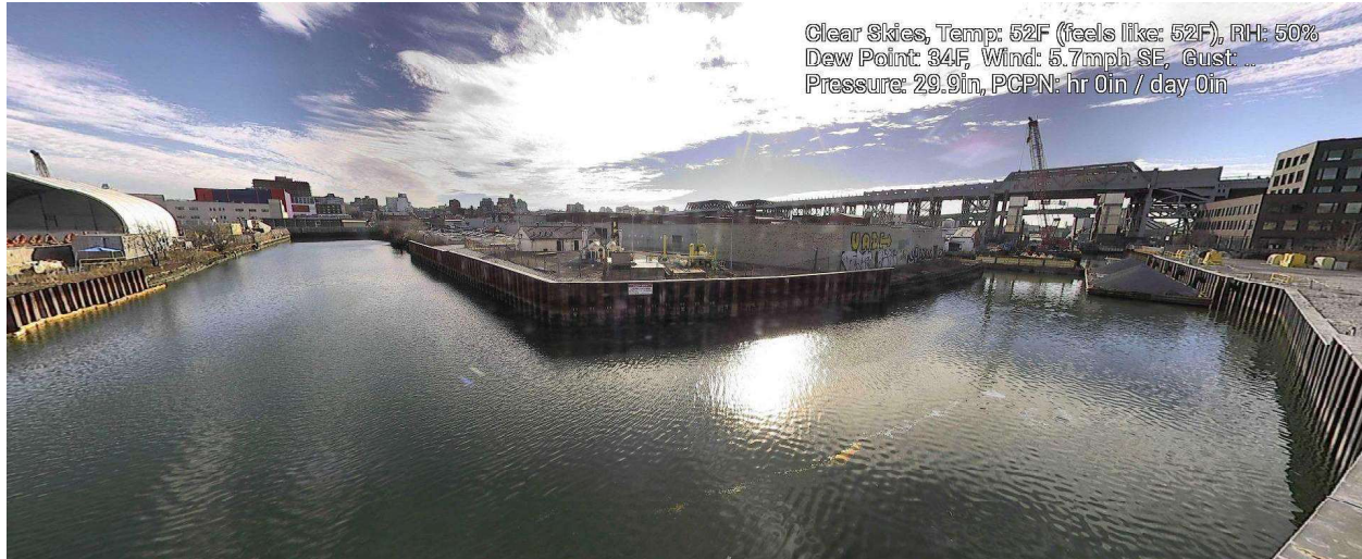
Figure 7 – December 31, 2024. General Conditions in Canal north of 9 th Street Bridge during in-waterway construction activities.
