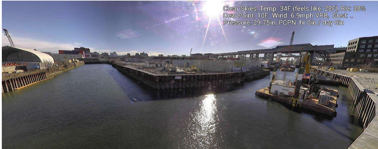
Figure 10 – January 9, 2025. General Conditions in Canal north of 9 th Street Bridge near TB6 during in-waterway construction activities.
