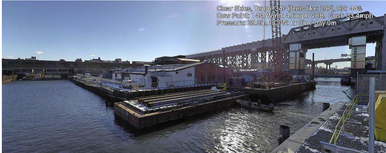
Figure 8 – January 7, 2024. General Conditions in Canal north of 9 th Street Bridge during in-waterway construction activities.
