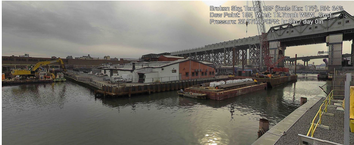
Figure 10 – January 16, 2025. General Conditions in Canal north of 9 th Street Bridge near TB6 during in-waterway construction activities.
