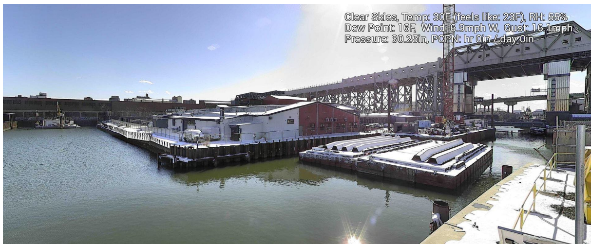
Figure 9 – January 20, 2025. General Conditions in Canal north of 9 th Street Bridge near TB6 during in-waterway construction activities.
