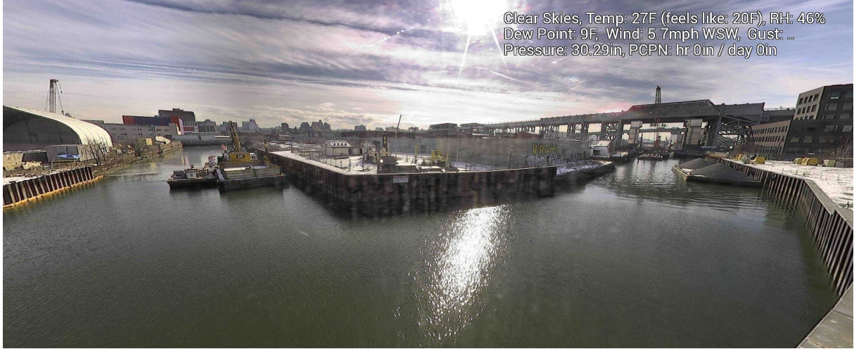
Figure 10 – January 23, 2025. General Conditions in Canal north of 9 th Street Bridge near TB6 during in-waterway construction activities.
