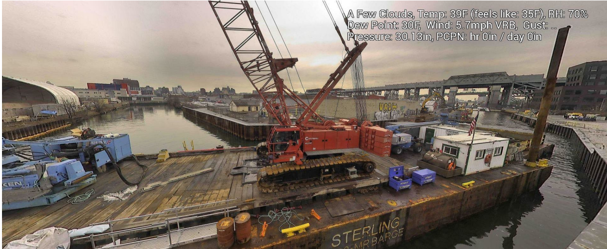
Figure 8 – February 3, 2025. General Conditions in Canal north of 9 th Street Bridge near TB6 during in-waterway construction activities.
