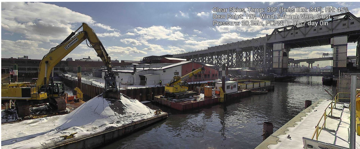
Figure 9 – February 10, 2025. General Conditions in Canal north of 9 th Street Bridge near TB7 during in-waterway construction activities.
