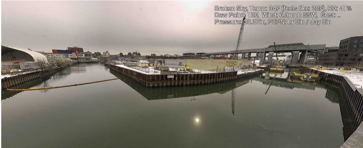
Figure 8 – February 11, 2025. General Conditions in Canal north of 9 th Street Bridge near TB6 during in-waterway construction activities.
