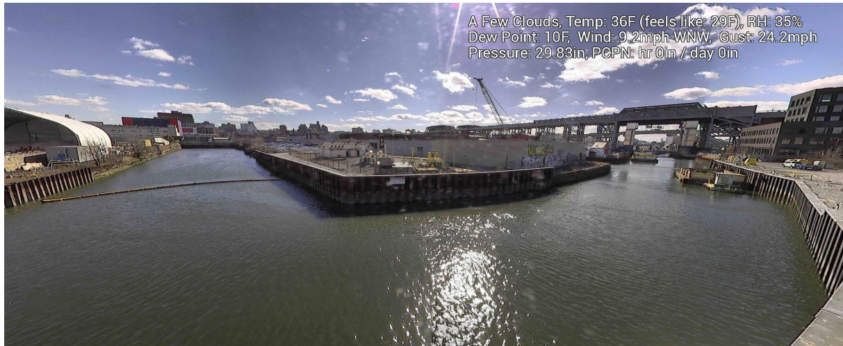
Figure 7 – February 17, 2025. General Conditions in Canal north of 9 th Street Bridge near TB6 during in-waterway construction activities.
