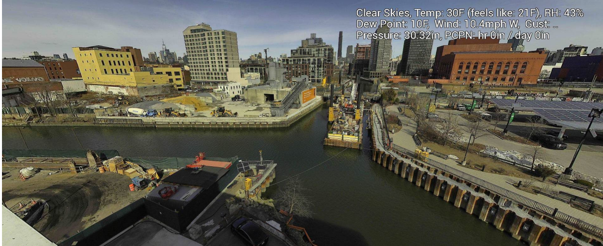
Figure 9 – February 19, 2025. General Conditions in Canal south of 3 rd Street Bridge near TB4 during in-waterway construction activities.
