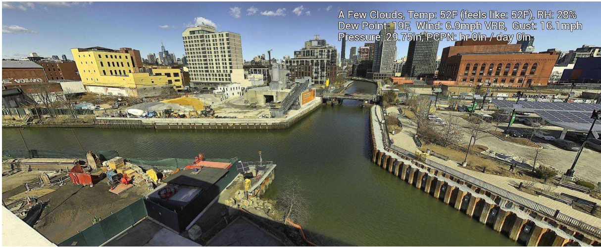
Figure 10 – February 28, 2025. General Conditions in Canal south of 3 rd Street Bridge near TB4 during in-waterway construction activities.
