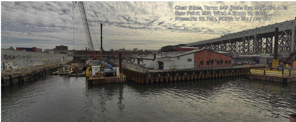
Figure 8 – February 25, 2025. General Conditions in Canal north of 9 th Street Bridge near TB6 during in-waterway construction activities.
