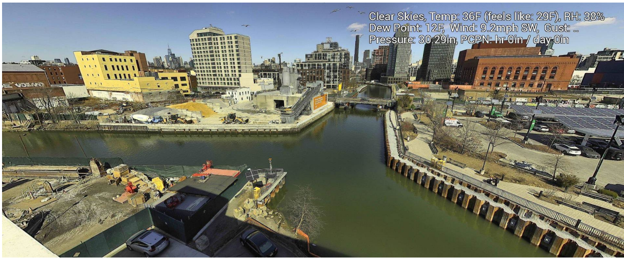
Figure 10 – March 3, 2025. General Conditions in Canal south of 3 rd Street Bridge near TB4 during in-waterway construction activities.
