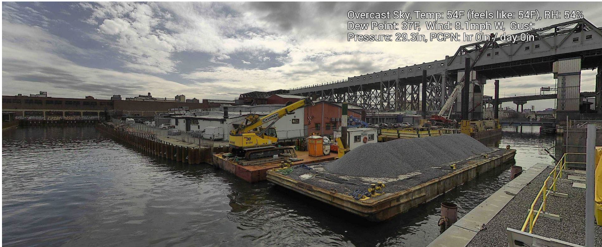
Figure 8 – March 6, 2025. General Conditions in Canal north of 9 th Street Bridge near TB6 during in-waterway construction activities.
