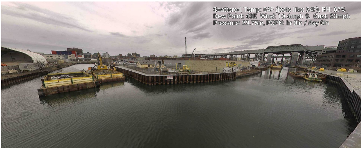
Figure 9 – March 5, 2025. General Conditions in Canal north of 9 th Street Bridge near TB6 during in-waterway construction activities.
