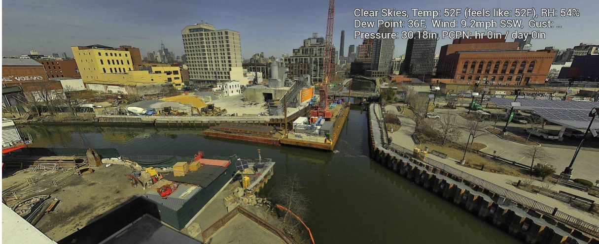
Figure 10 – March 14, 2025. General Conditions in Canal south of 3 rd Street Bridge near TB4 during in-waterway construction activities.
