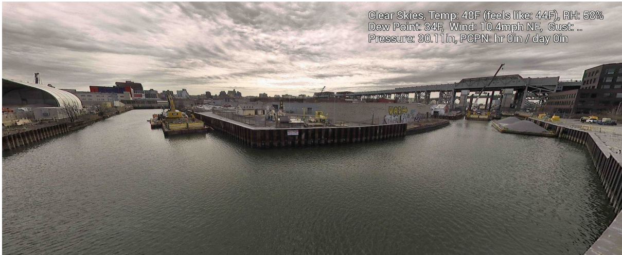
Figure 9 – March 13, 2025. General Conditions in Canal north of 9 th Street Bridge near TB6 during in-waterway construction activities.
