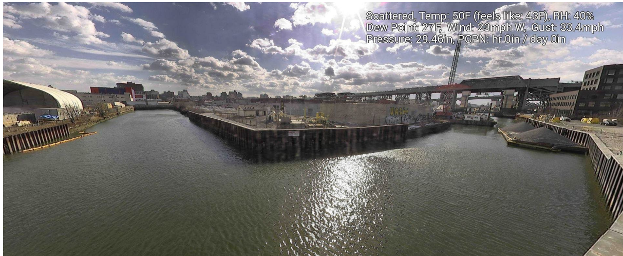
Figure 8 – January 29, 2025. General Conditions in Canal north of 9 th Street Bridge during in-waterway construction activities.
