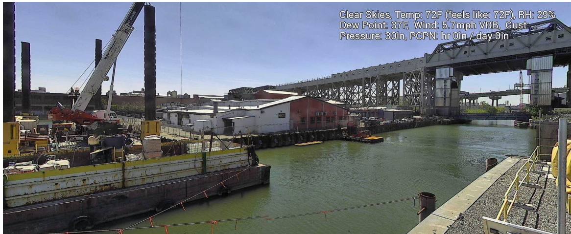
Figure 9 – April 30, 2025. General Conditions in Canal north of 9 th Street Bridge near TB6 during in-waterway construction activities.
