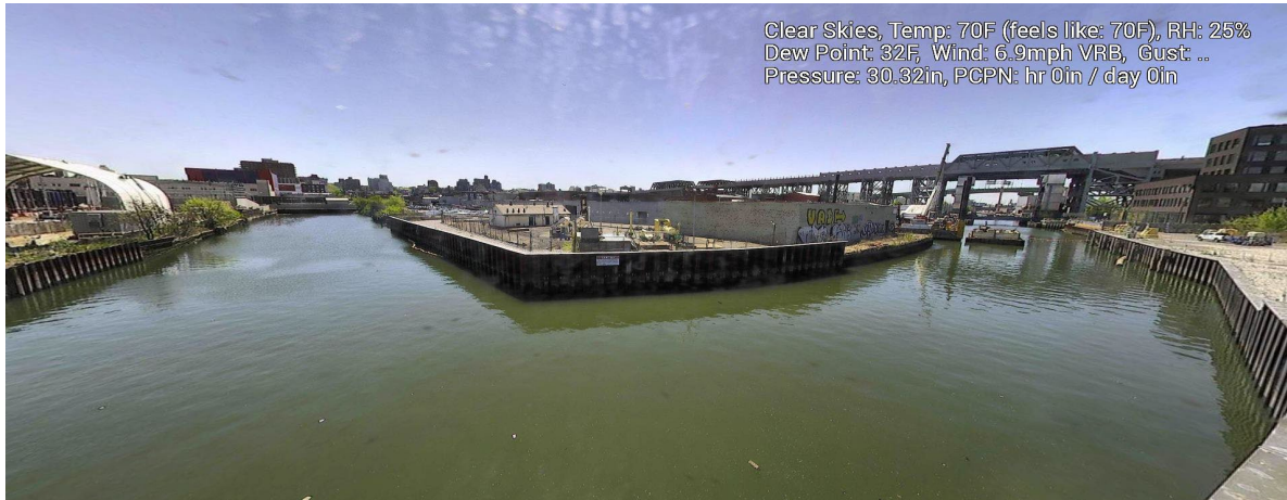
Figure 8 – April 28, 2025. General Conditions in Canal north of 9 th Street Bridge near TB6 during in-waterway construction activities.
