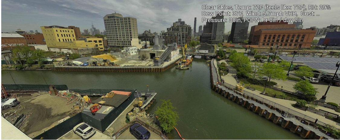
Figure 10 – May 2, 2025. General Conditions in Canal south of 3 rd Street Bridge near TB4 during in-waterway construction activities.
