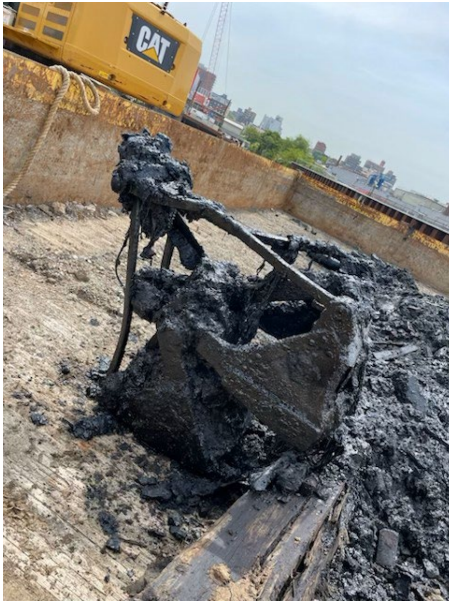
Photograph 1. Initial condition of the bucket from Turning Basin 6 (Chris Sheedy, May 27, 2025).
